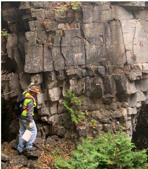
BEFORE GRAFFITI REMOVAL
